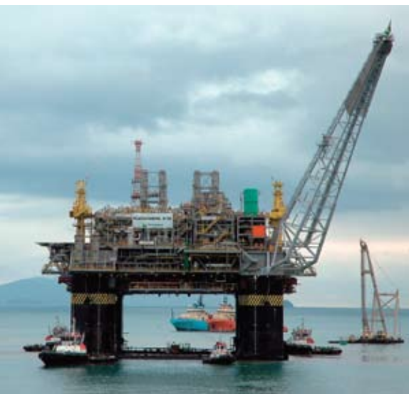
Teamwork and experience enabled the BrasFELS team to successfully complete marine mating operations for the FPU P-56 within a tight timeframe of 13 days
