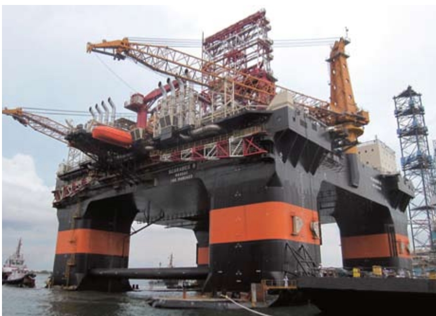
Saipem's Frigstad D90 semisubmersible rig, Scarabeo 9, has arrived at Keppel FELS' Singapore yard for completion work
