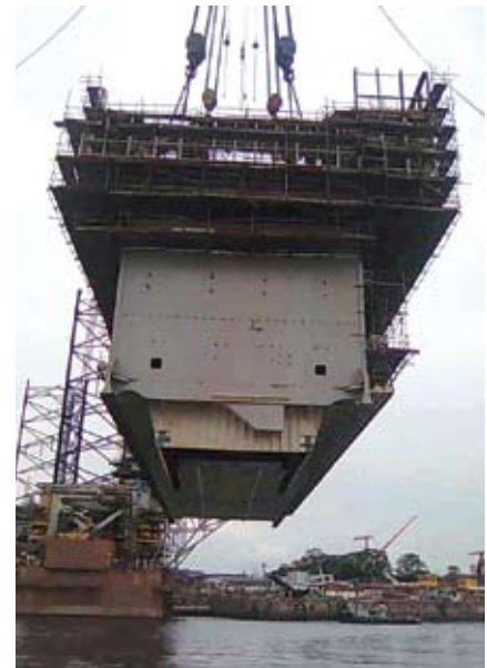
Under the Asian Lift crane operator's experienced hands, the lifting job was completed safely, swiftly and with precision
