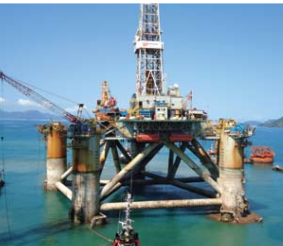
Repeat customer QGOG brings another semisubmersible drilling rig, Atlantic Star, to BrasFELS for repair and upgrading works
